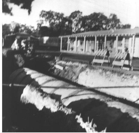
Pipe laid in trench. The building in the background was in the BV Trailer Park. Fall 1958.
