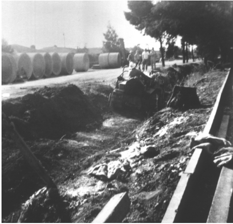
Deepening the creek channel to enable emplacement of the culvert alongside the Buena Vista Trailer Park, Fall 1958.
