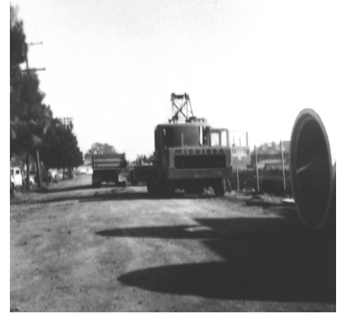
Excavation machinery on Los Robles by the McElroy Lumber Yard across from the BV. Fall 1958.
